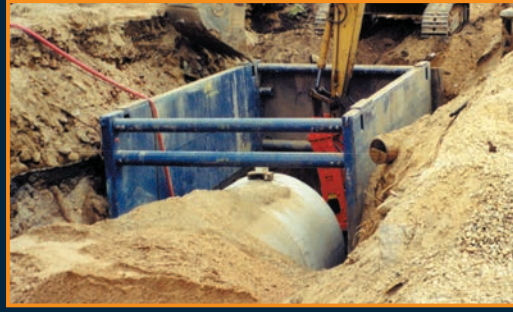
Steel Trench Shield
